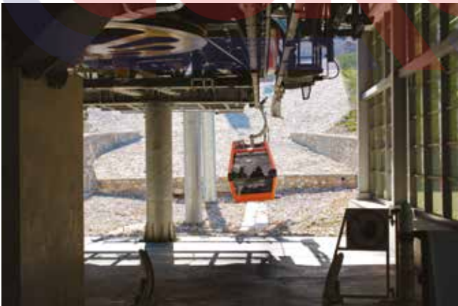
Locking the drive pulley of a cable car using SIT-LOCK® 4.
